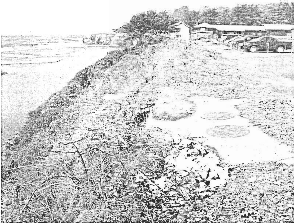
Photo 5. Exposed traffic slab covering interceptor tank due to eroding fill.
